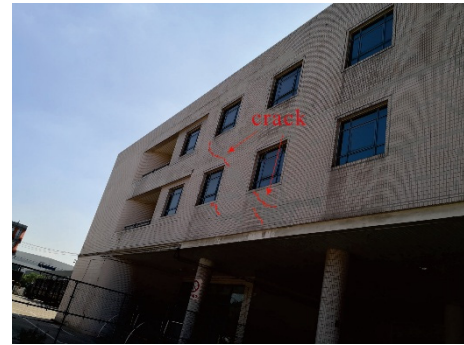
The wall of SF Express company is cracked
