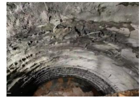
First lining failure
