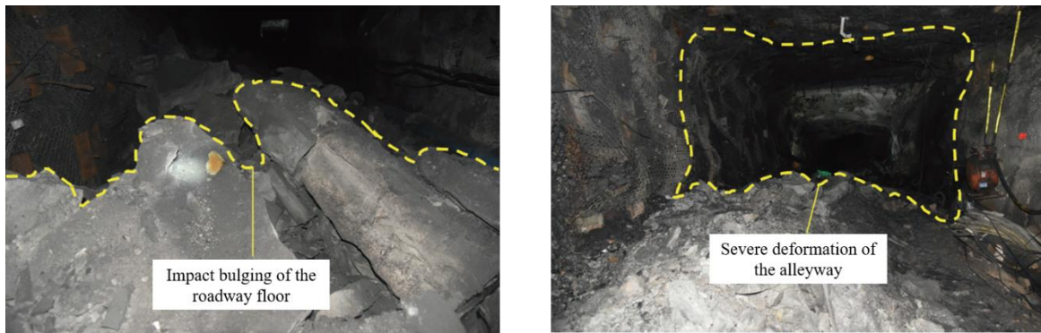
Fig. 4 Large deformation of gateroad caused by strong mining pressure
