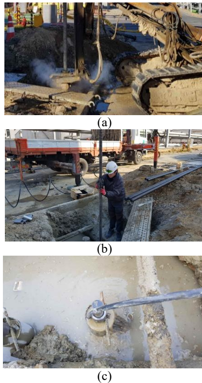
Fig. 4 Construction of micropile : (a) ground boring, (b) insertion of casing and steel bar, and (c) grouting in the bored hole
