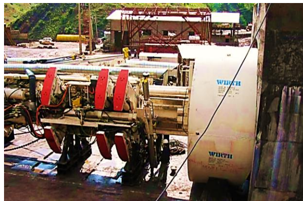
Fig. 5 Open gripper TBM manufactured by Wirth
