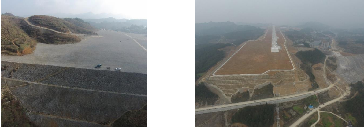
(a) During construction of the high rockfill embankment (b) After the construction of the runway Fig. 10 Aerial view of the Maotai Airport embankment from unmanned drone
