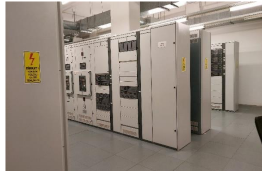
Fig. 16 EnerjiSA Üretim Bandırma-I NG CCPP, Control Building Low Voltage Room
