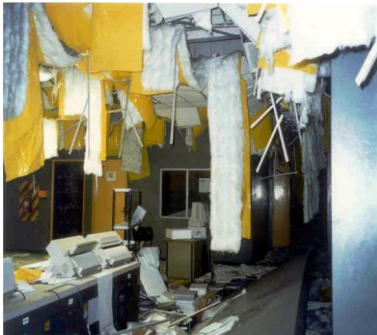
(a) 8.4 magnitude Peru Earthquake, 2001; Suspended ceiling, lighting, insulation damages in the Industrial Plant Control Building
