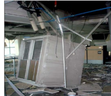
(c) 8.8 Magnitude Chile Earthquake, 2010; HVAC equipment damage in Santiago Airport Terminal Building
