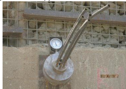
(c) Close-up of a load cell
