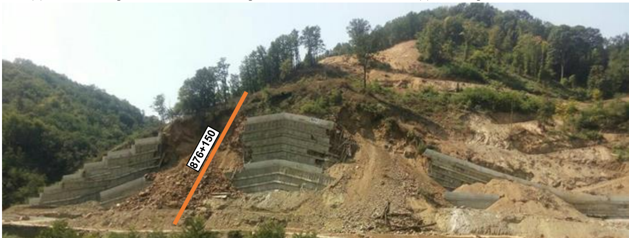
(d) Failure of cut no. 2 in August 2018 (orange line indicates position of cross-section 876+150)
