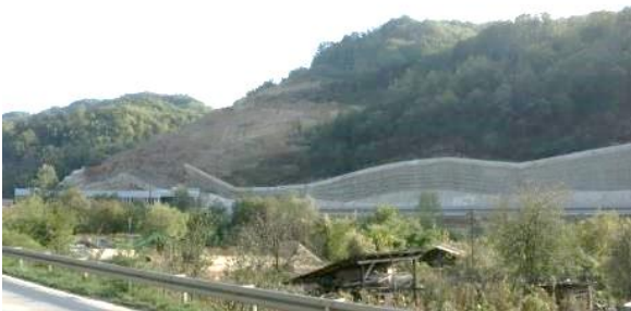
(c) View of the failed section after removal of unstable material and slope rearrangement
