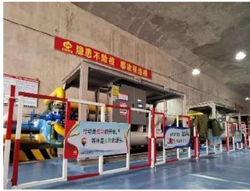
(a) Equipments for freezing
