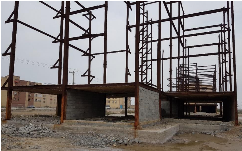
Fig. 14 Five-story buildings constructed across the area of the project with no evidence of excessive settlements during the past 20 years
