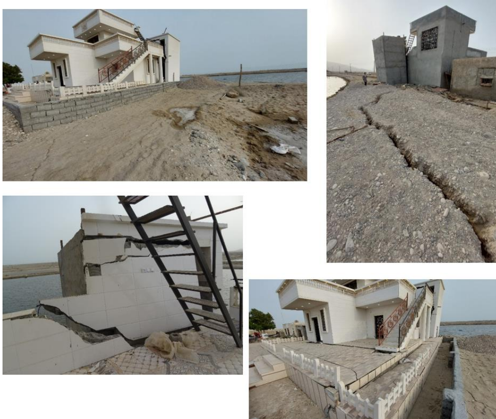
Fig. 29 A damaged building that could not tolerate excessive settlement
