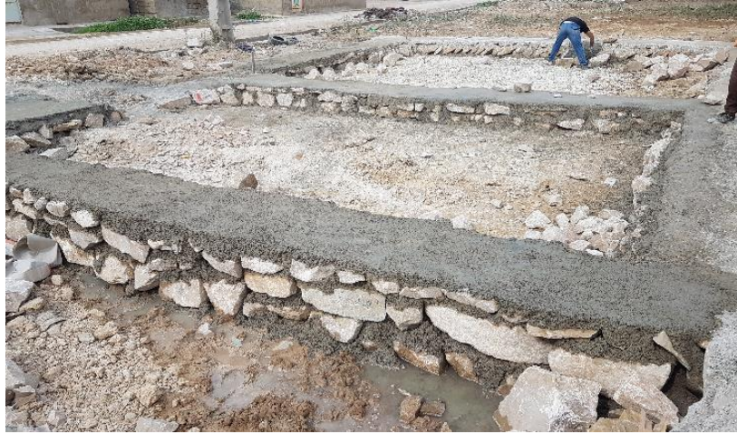
Fig. 13 Typical subgrade construction on the site consisting of stone mixed with lime mortar
