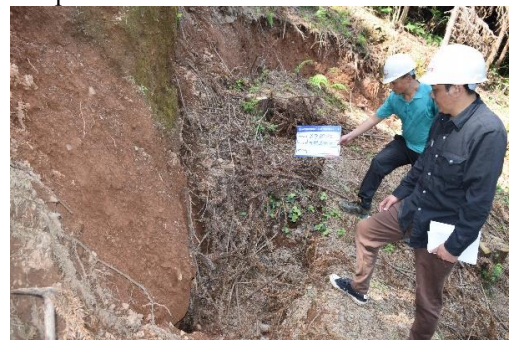
(c) Tensile cracks at the trailing edge of the slope
