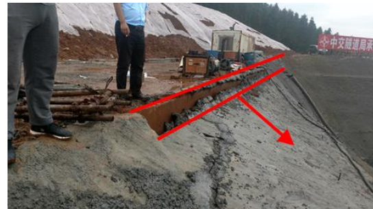
(b) Slope cracking
