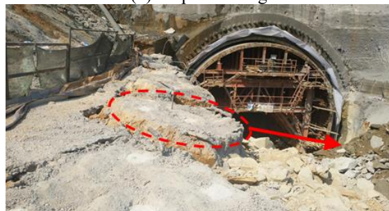
(c) Lateral displacement of pile top
