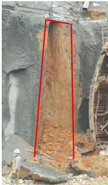
(a) Collapse of the soil between piles
