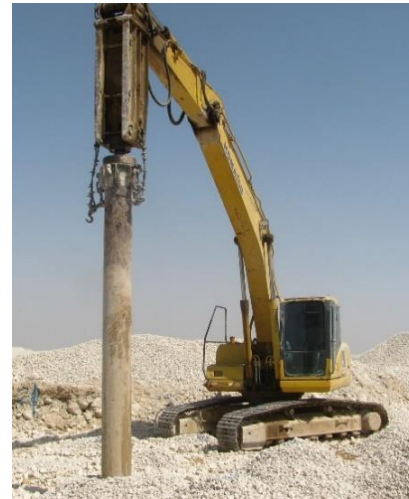
Fig. 3 Hammering the shuttle into the soil through the shuttle hammer mounted on the hydraulic hammer
