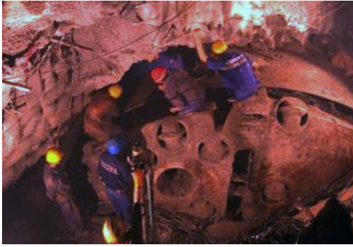
Fig. 1 TBM tunnel collapse
