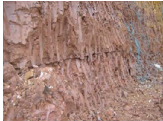
Fig. 1 The natural expansive soil in the foundation pit of the East Huada Square
