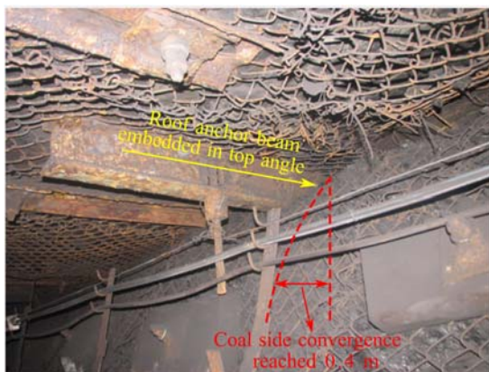
Fig. 1 The roof anchor cable embedded in the roadway top angle affected by coal pillar convergence deformation
