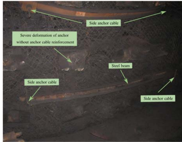
Fig. 11 Effect diagram of anchor cable reinforcement in the section coal pillar side
