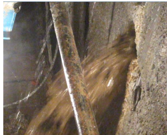
Fig. 2 Photo of the gushing water and sand from shaft side wall
