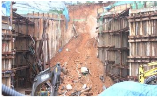
Fig. 2 Collapse of convex corner in deep excavation
