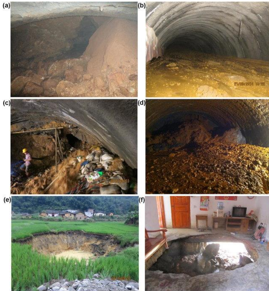
Fig. 1 A number of hazards that tunnels face due to unfavorable geological conditions (Yuan et al. 2019)
