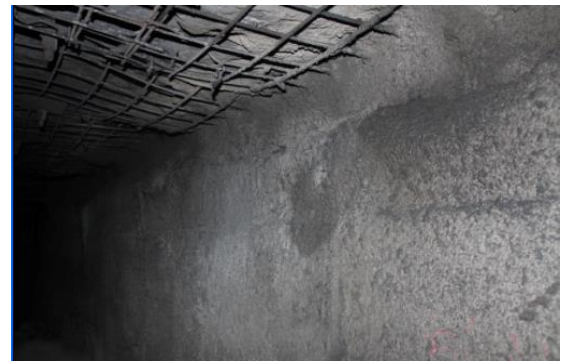
Fig. 11 Photo of the roof-contacted filling by side of gas laneway (tunnelling direction)
