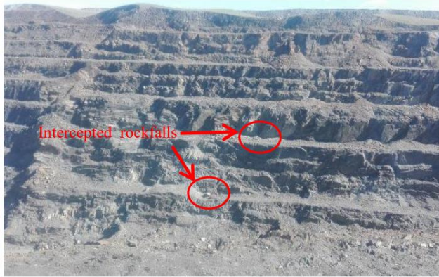
Fig.15 Interception effect of a platform paved with a gravel cushion for rockfall disasters
