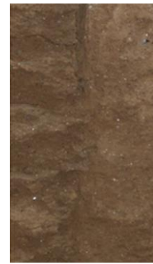
(b) Lateral crack of D-1
