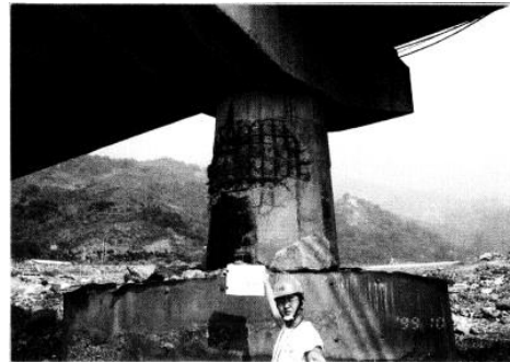
(b) Pier damage of the Chang-Qing Bridge
