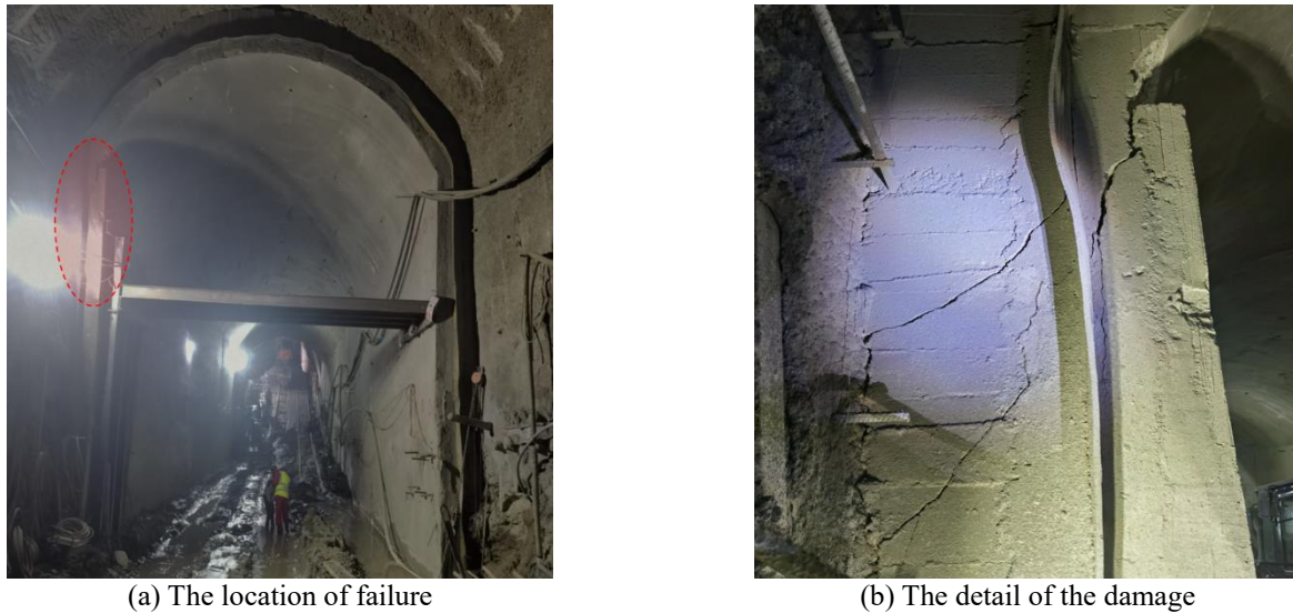
Fig. 11 Failure of construction tunnel lining in the intersection area
