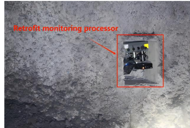
Fig. 9 Retrofit monitoring processor
