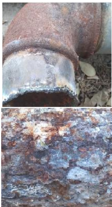
Fig. 1 Biological corrosion of pipes buried in the soil
