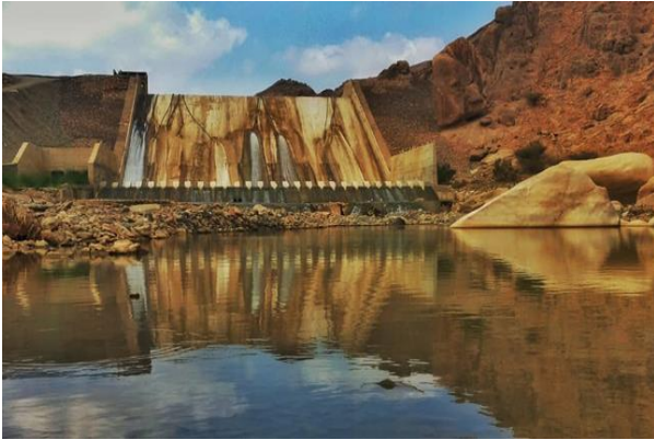
Fig. 32 UG Dam 1 (Siphon system on spillway due to gates were closed as a result of the rise of the silt)
