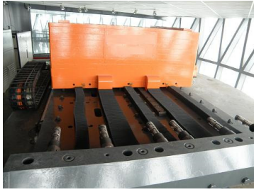
Fig. 17 Photograph of AMD in Canton Tower
