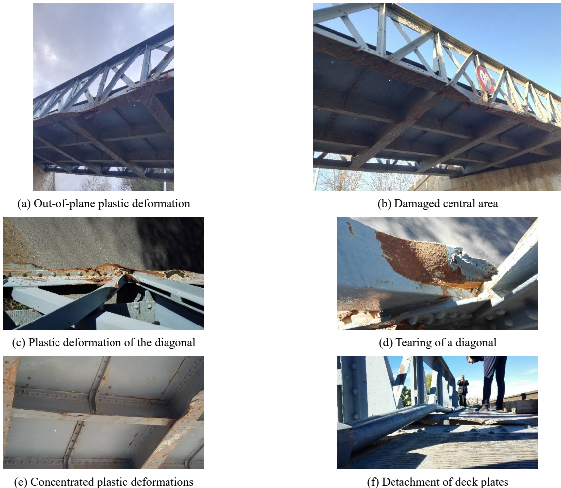
Fig. 3 Pathologies identified on the structure
