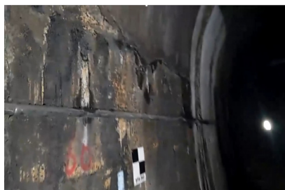
(a) Walk toward damage
