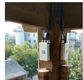
(b) FBG inclination sensor on the cantilever column
