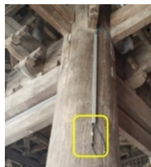
(a) FBG strain sensor on the top of the column
