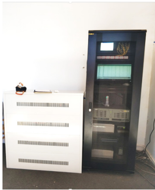
Fig. 15 Cabinet in the monitoring center
