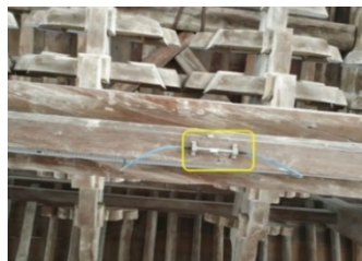
(b) FBG strain sensor on the mid-span of the beam
