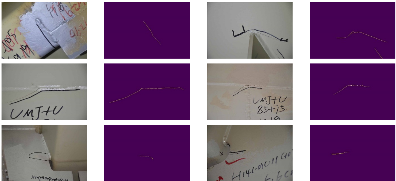
Fig. 8 A few representative original images and binary annotations for tiny cracks
