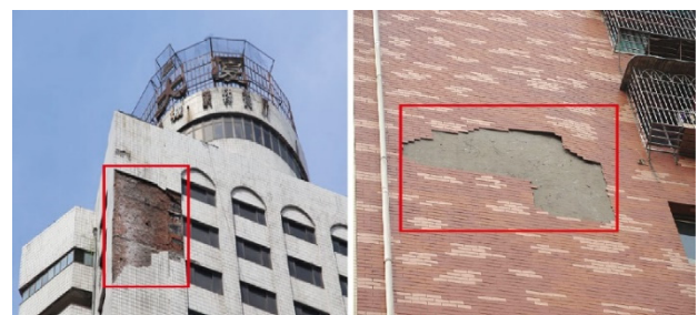
Fig. 1 Debonding defects of BDLs
