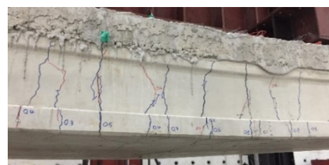
(b) Cracks of M-550
