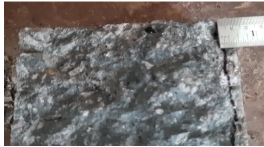
Fig. 11 The crack in unreinforced specimen 500 μm in concrete type 2
