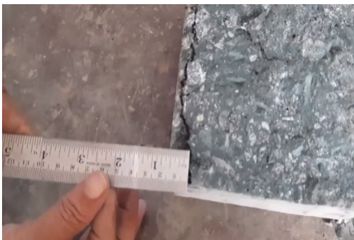
Fig. 10 Measuring the crack in samples
