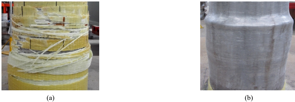
Fig. 15 Typical damage modes of FRP composite and steel tube: (a) fractured and de-bonded GFRP; and (b) buckled steel tubes
