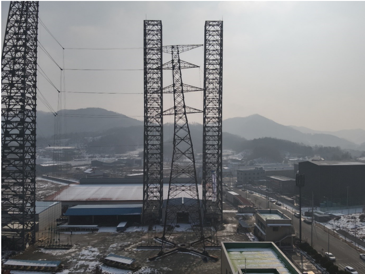
(a) Failure of tower overview
