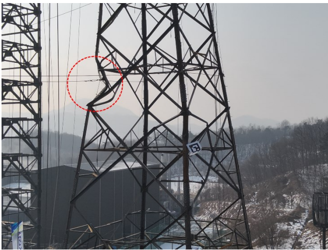
(b) Failure mode at s7
