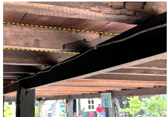
Fig. 1 Scarf joint in floor structure on Nuwo Sesat, traditional building in Indonesia
